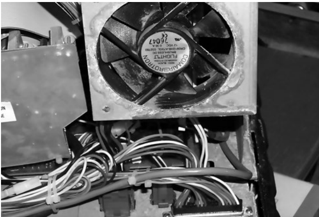
FIGURE 15.2 Corrosion of a fan bracket.
